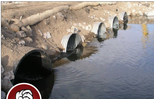
Fig. 5-5. Riprap with no fines should be installed at the approach to prevent sediment from entering the stream. If temporary, a silt fence could be used with sand bags anchoring the fabric on the culverts.
