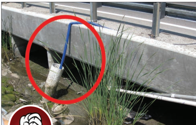
Fig. 3-18. Direct discharge from dewatering operations into bridge crossings or gutter areas can allow pollutants to enter into streams and rivers.
