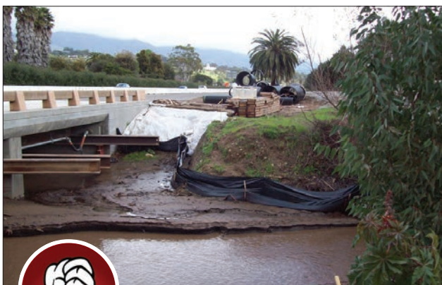
Fig. 3-12. This picture shows an improperly installed silt fence (trenching, post and fence placement). This is a common problem with some bridge projects and limited work area. Silt fence backing or reinforced silt fence is recommended.
