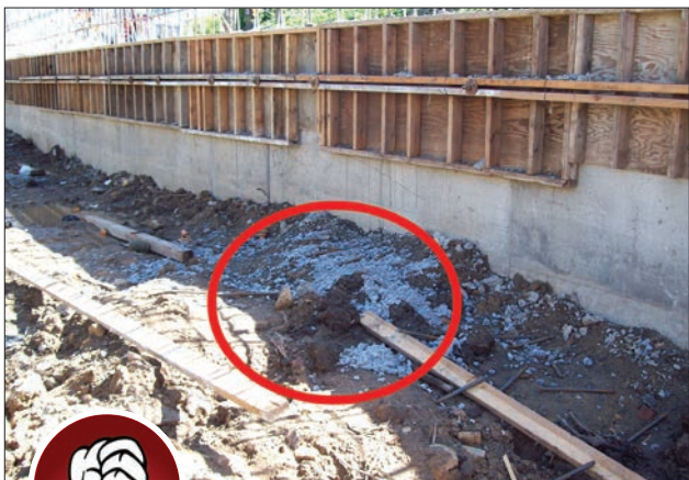
Fig. 2-14. This picture depicts residue from cleanout of a concrete truck not performed in a controlled washout area.
