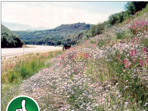
Fig. 1-2. Construction sites should aim to produce no more sediment risk than the natural condition as this re-vegetated slope does.
