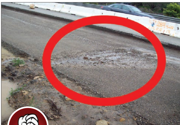
Fig. 2-6. Careful inspection could have prevented this spill onto the roadway. Stormwater inlets near the areas should immediately be assessed for impact. Since the spill appears small, rags may prove effective for cleanup.
