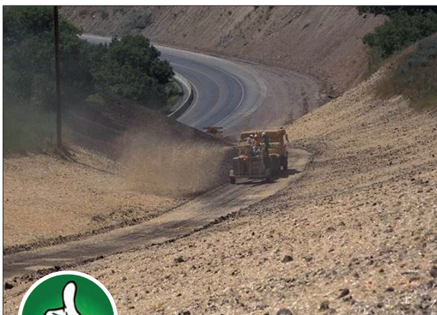
Fig. 4-10. Hydraulically applied straw mulch is an effective means to anchor temporary or permanent seeding to a highway slope.
