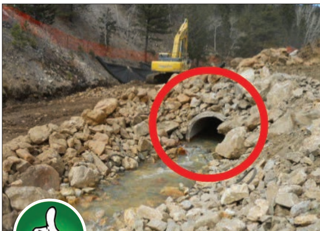
Fig. 5-4. This is a good application of a temporary culvert. Note the riprap approach to the culvert. Source: Colorado DOT
