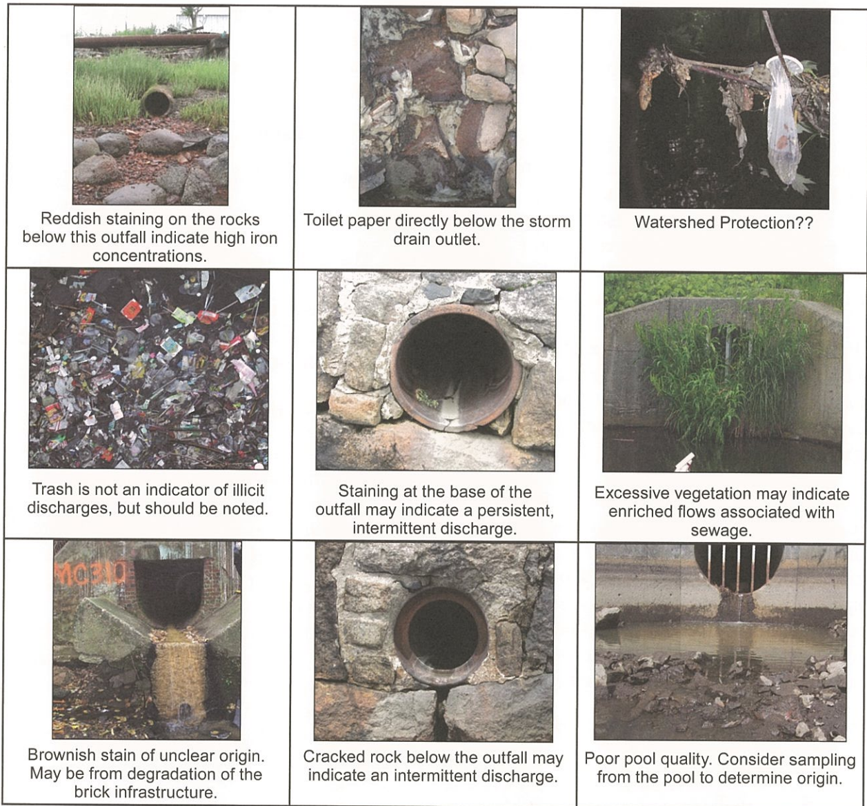
Figure 39: Typical Findings at Both Flowing and Non-Flowing Outfalls
