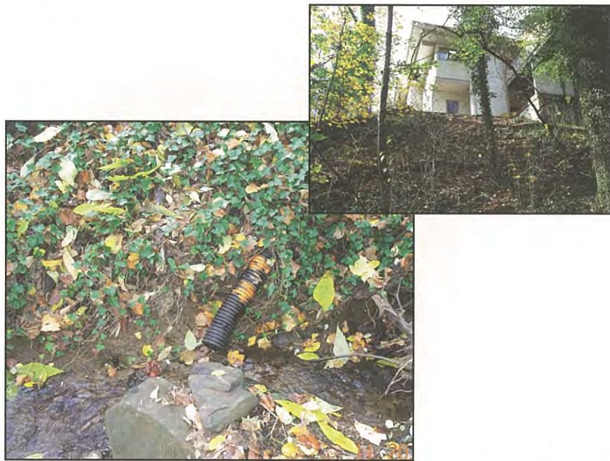
Figure 25: The origin of this corrugated plastic pipe was determined to be a roof leader from the house up the hill.
