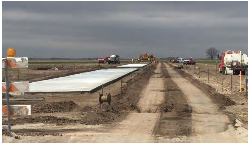
New Northwest Third Addition paving began March 30. The photo above shows Patriot Drive extension.
