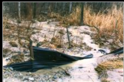
Failed silt fence
